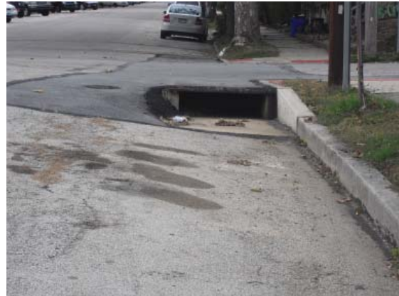
Current gutter condition
